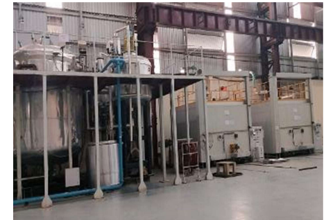
VPI Plant with Oven
